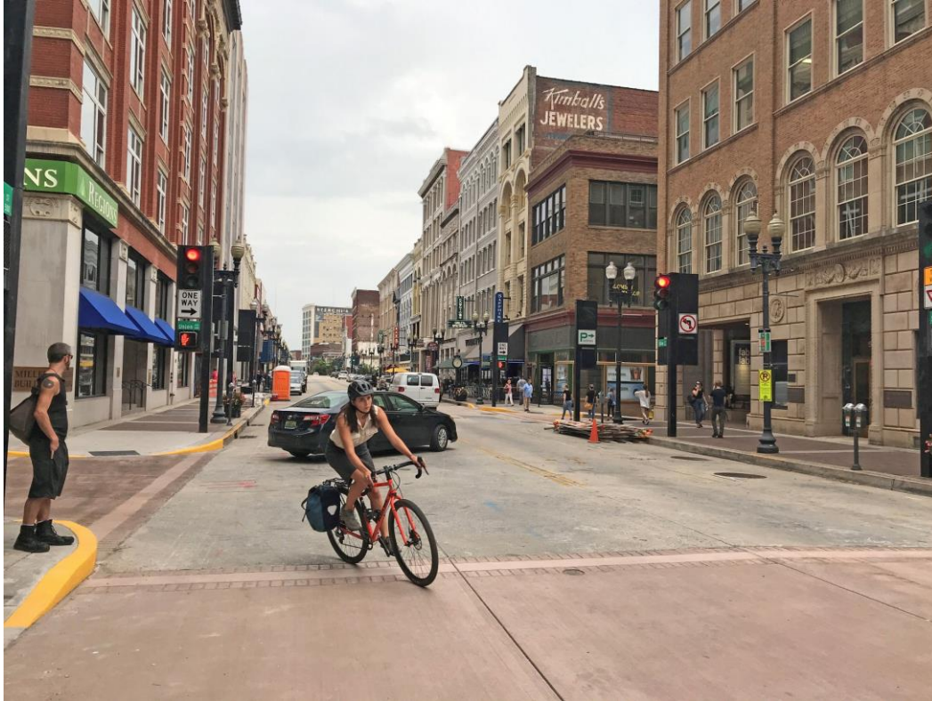
Looking North at finished crosswalks at S Gay Street and Union Avenue August 2018
