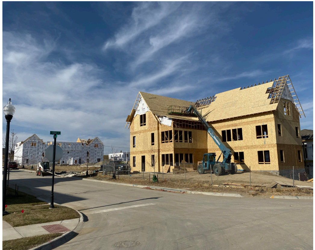
Figure 2.4 The simple forms, smaller size, and compatibility with wood-frame construction help maximize affordability and investment returns, and are consistent with the construction strategies familiar to most residential homebuilders, as shown in this under-construction MMH project in Papillion, Nebraska.
