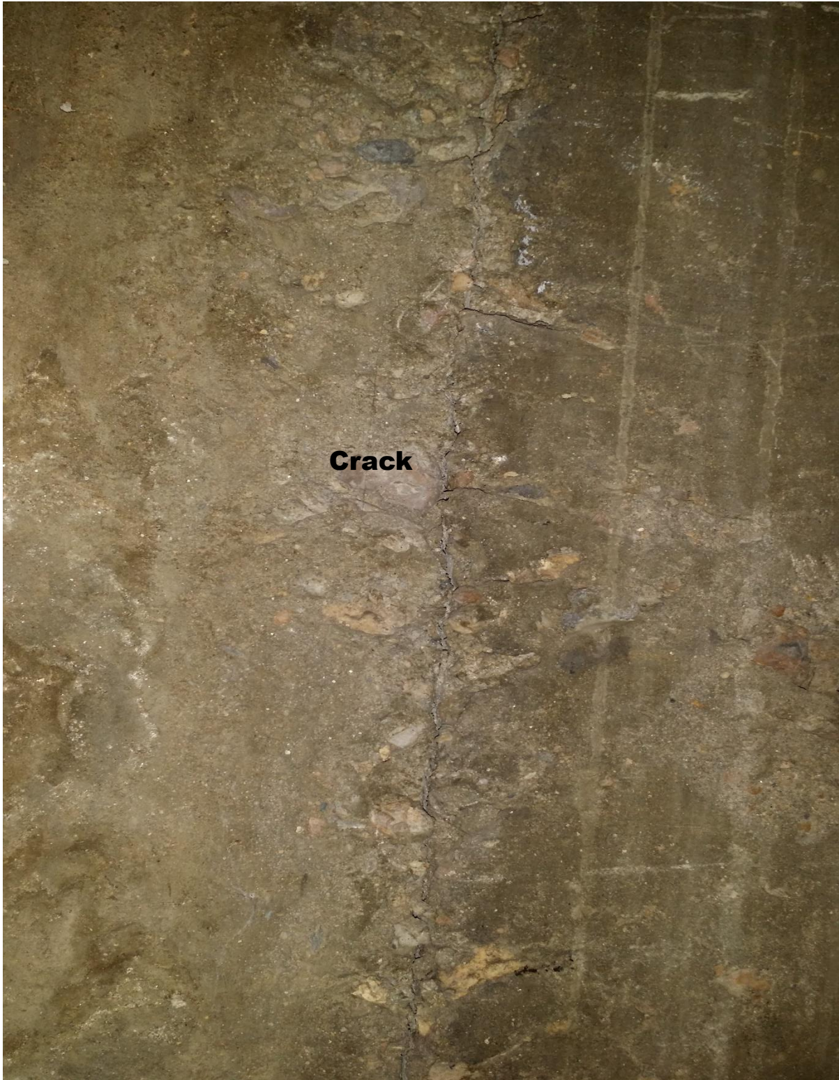
Mechanical Room2 Floor
