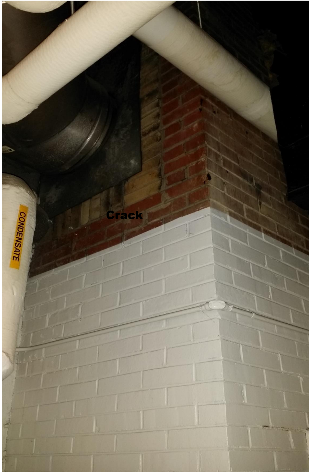
Chimney in Boiler Room
