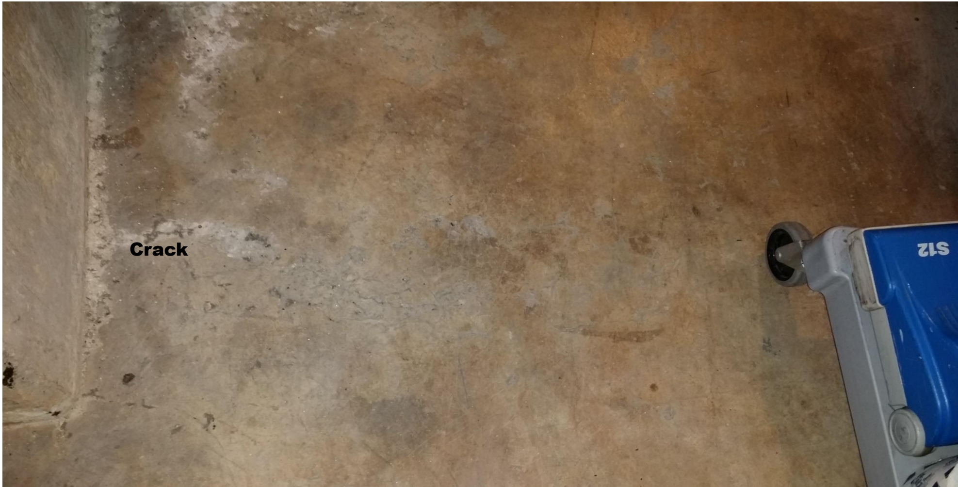
Electrical Closet Floor
