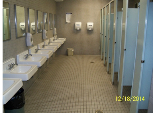
P.10 Plumbing fixtures – women's restrooms
