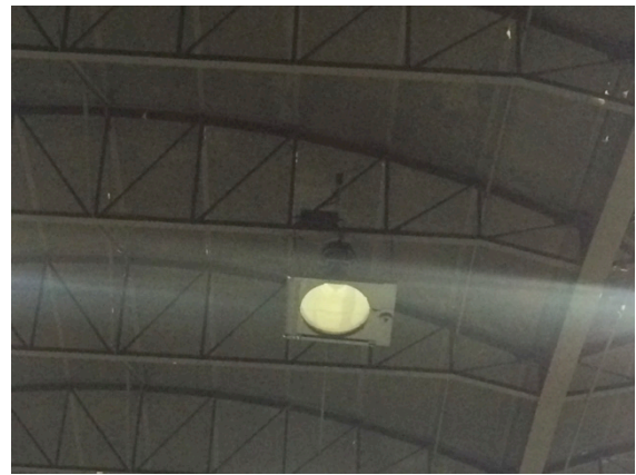
E.19 Sports Lighting for Coliseum
