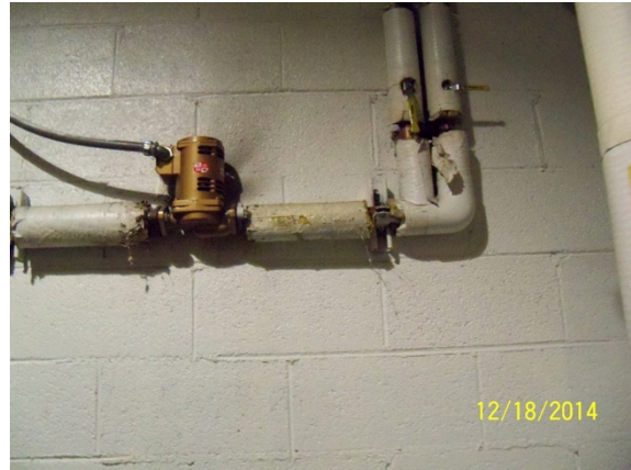
P.15 Hot water recirculation pump
