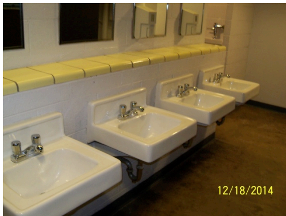
P.8a Plumbing fixtures – sinks
