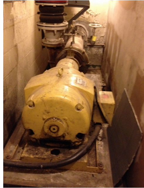
M.8 Condenser Water pump
