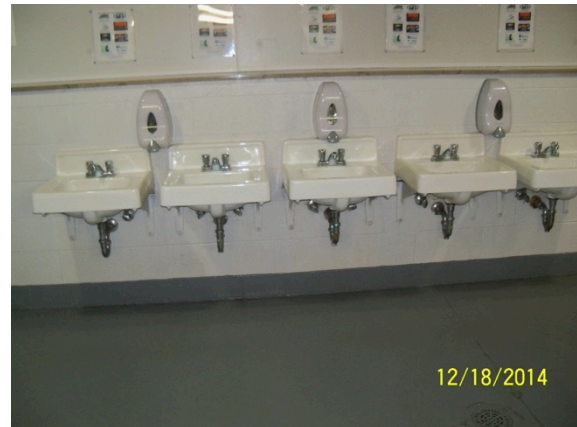
P.8b Plumbing fixtures - sinks
