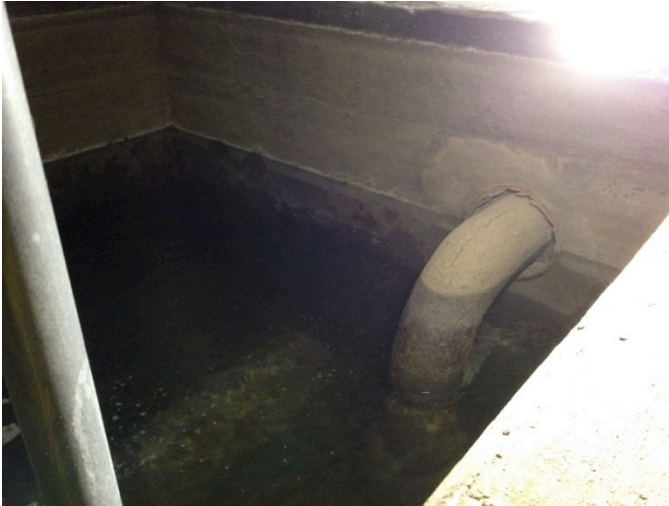
M.7 Condenser water basin
