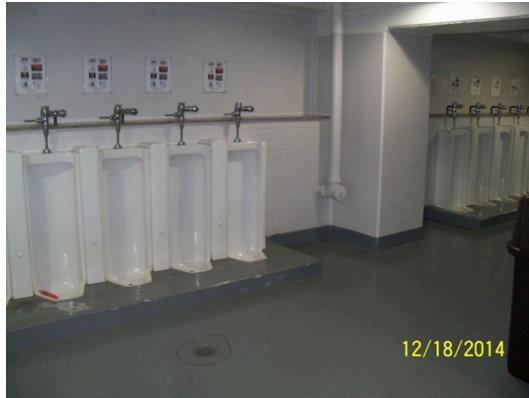
P.10 Plumbing fixtures – urinals
