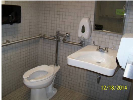
P.9 Plumbing fixtures – bathroom stall
