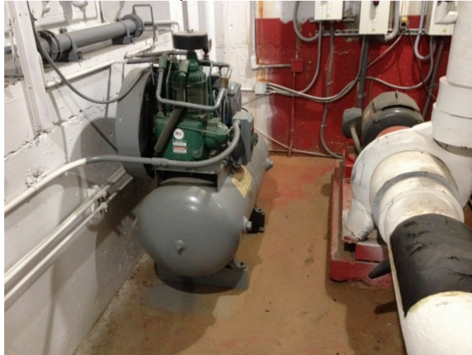
M.18 Control Air compressor
