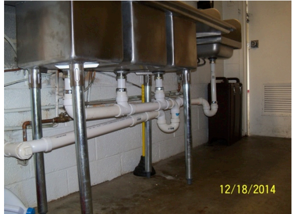
P.6 PVC waste piping
