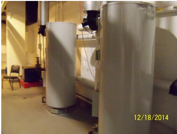
P.14 Gas water heaters
