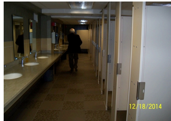
P.13 Plumbing fixtures - women's restroom, below level 2
