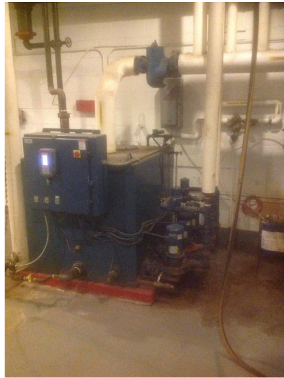
M.10 Steam condensate feed water pumps
