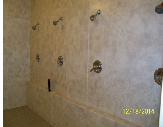
P.11 Plumbing fixtures – gang showers
