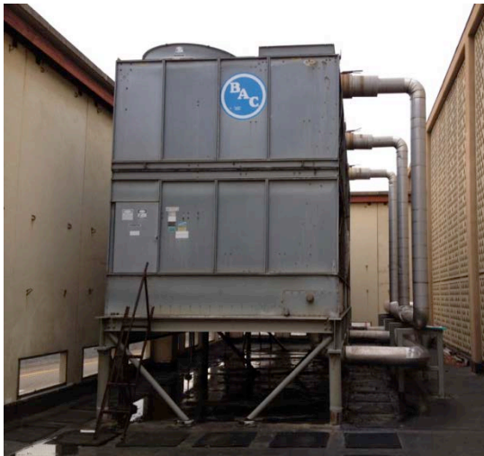
M.6 Cooling tower
