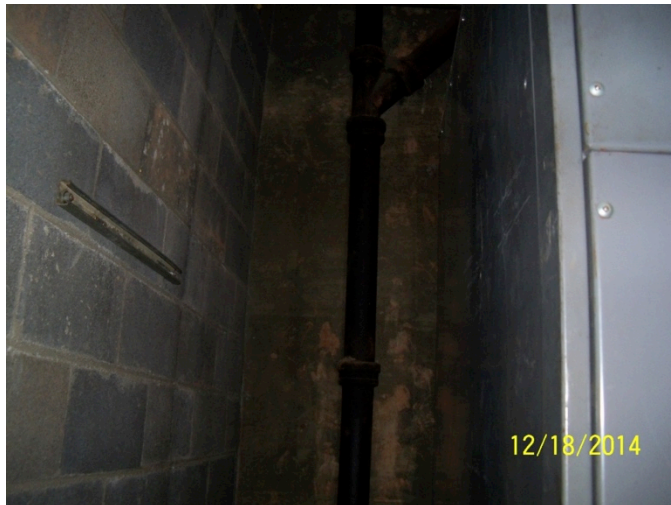
P.7 Bell and Spigot cast iron waste piping
