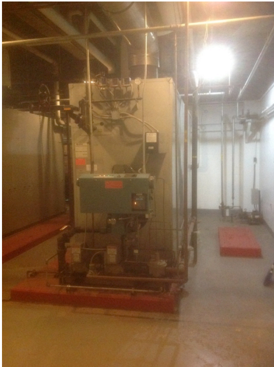
M.9 Steam boilers
