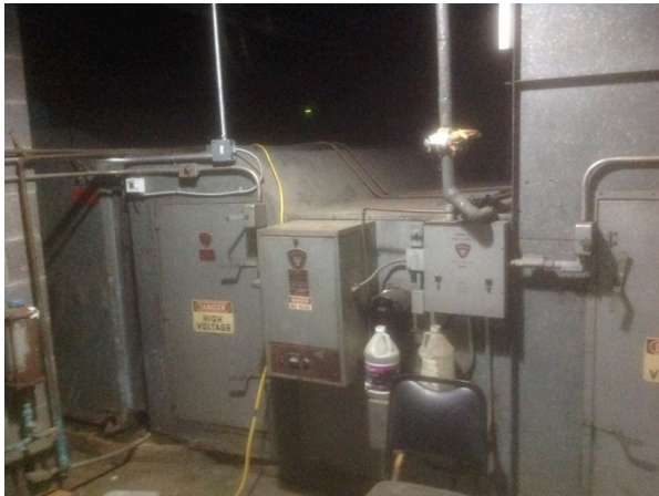
M.16 Auditorium stage AHU
