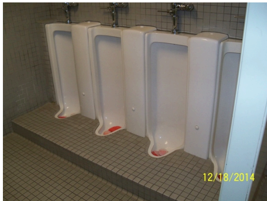
P.12 Plumbing fixtures – in floor urinals
