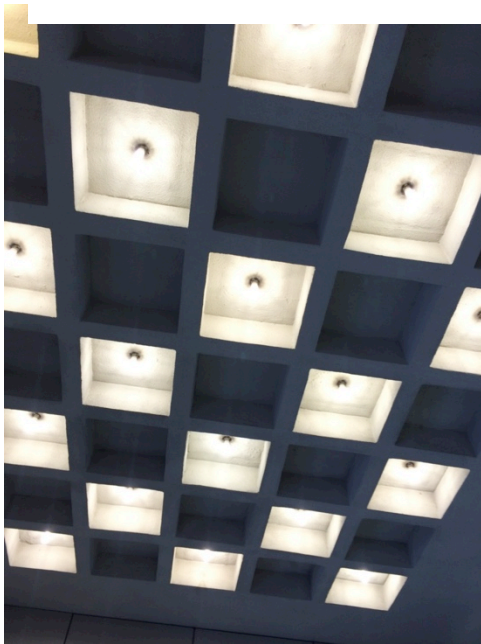
E.14 Incandescent lighting with Self Ballasted Fluorescent Lamps (Lobby)
