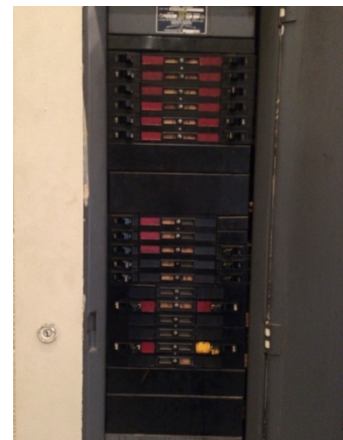
E.7. Electrical Panel cover not fitting properly.
