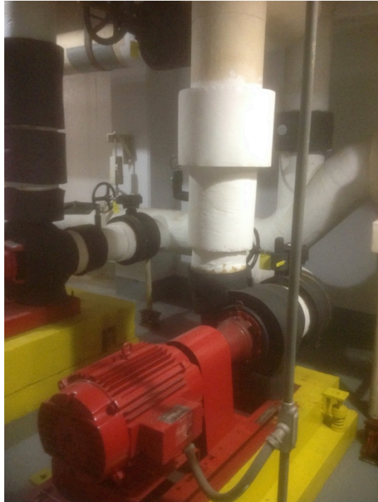
M.5 Chilled water pumps
