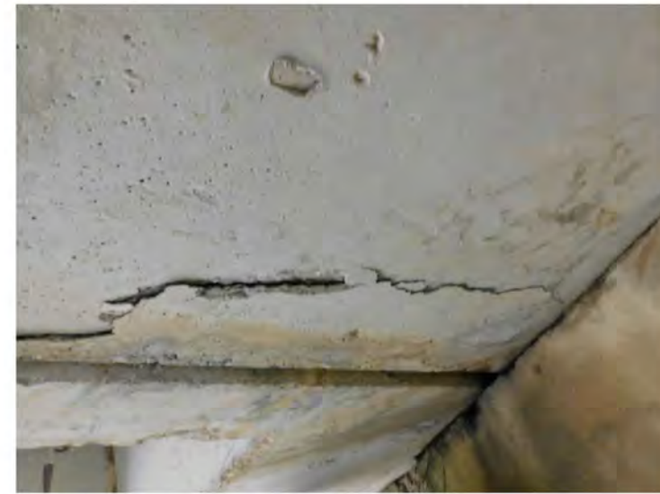
CRACKING BEAM D @ ABUTMENT 1
