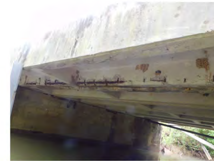
SPALLING W/ EXPOSED REBAR / UP TO 2" DEEP ALONG ENTIRE EDGE OF FLANGE / BEAM A (RT)
