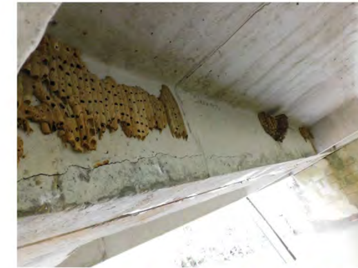
CRACKING / DELAMINATION / (LT) FLANGE BEAM B
