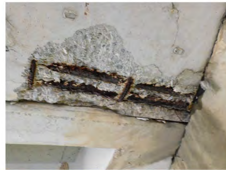
SPALL W/ EXPOSED REBAR (2'X1'X1/2") BEAM C @ ABUTMENT 1
