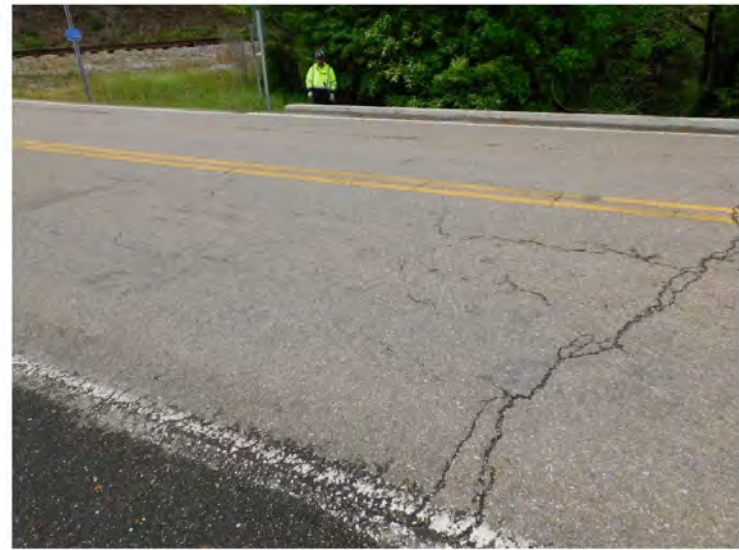
VIEW ACROSS DECK (NOTE: RAVELLING)
