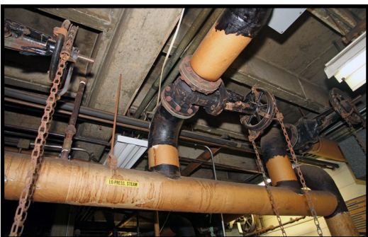
Original boiler system
