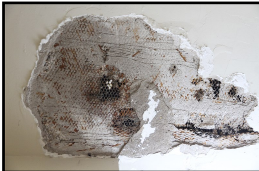
Water damage on ceiling
