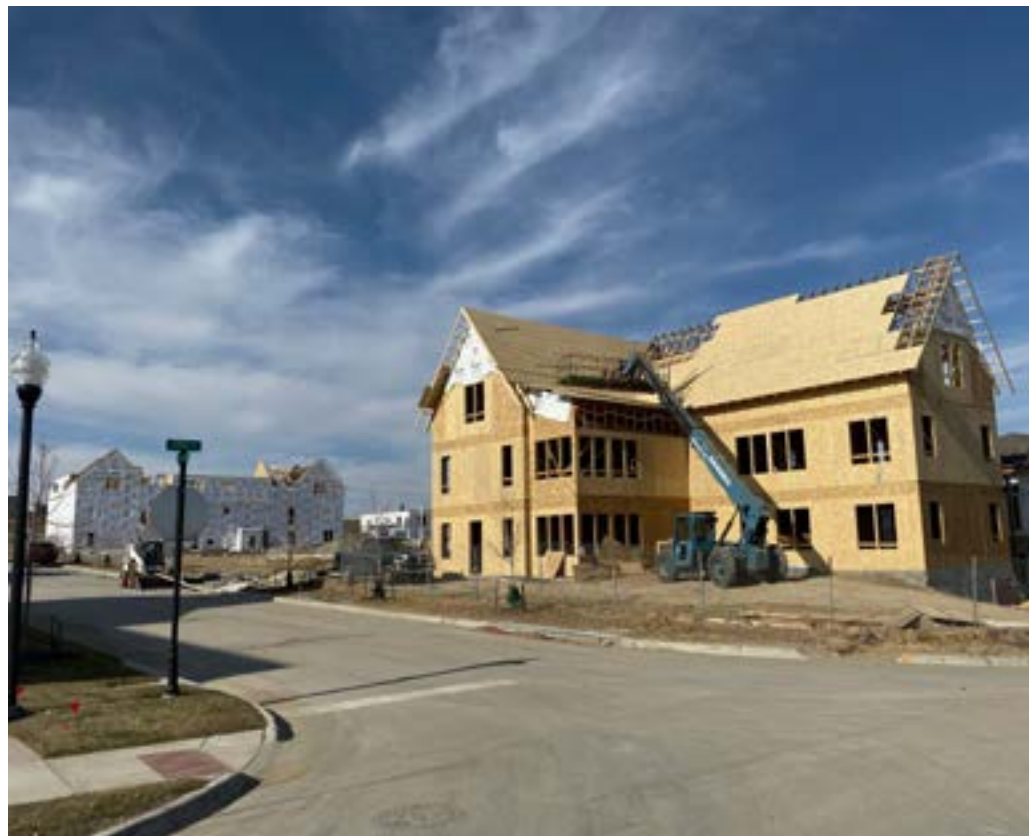
Figure 2.4 The simple forms, smaller size, and compatibility with wood-frame construction help maximize affordability and investment returns, and are consistent with the construction strategies familiar to most residential homebuilders, as shown in this under-construction MMH project in Papillion, Nebraska.
